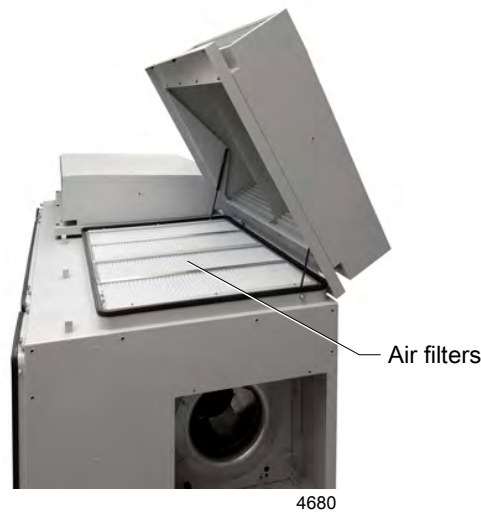
Figure 4-11. Air filter check
