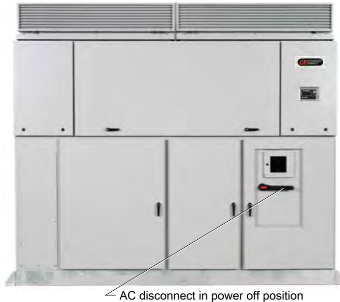
Figure 5-12. AC disconnect power OFF
